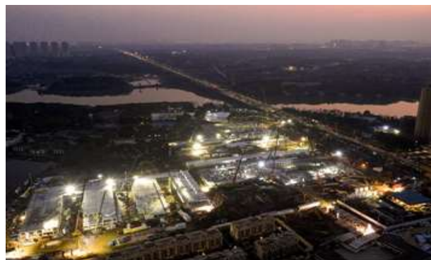
Figure 2 The use of drones hovering around 50metres above ground as a light source during the construction of hospital buildings in Wuhan, China (Source: Sharma, 2020)
